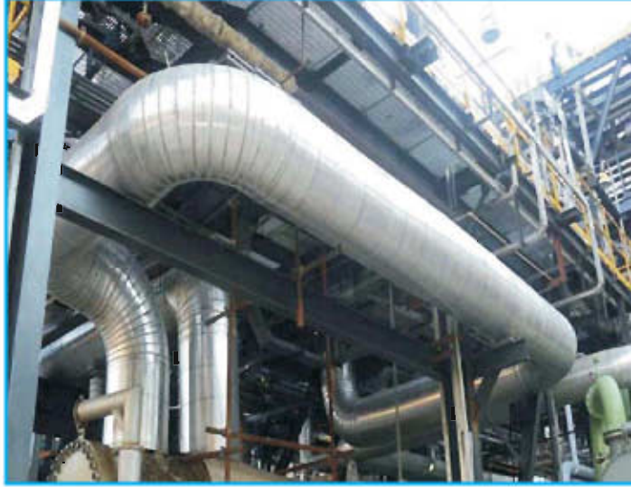
A View of Compressor Area : Piping Insulation at NFL Nangal project.
