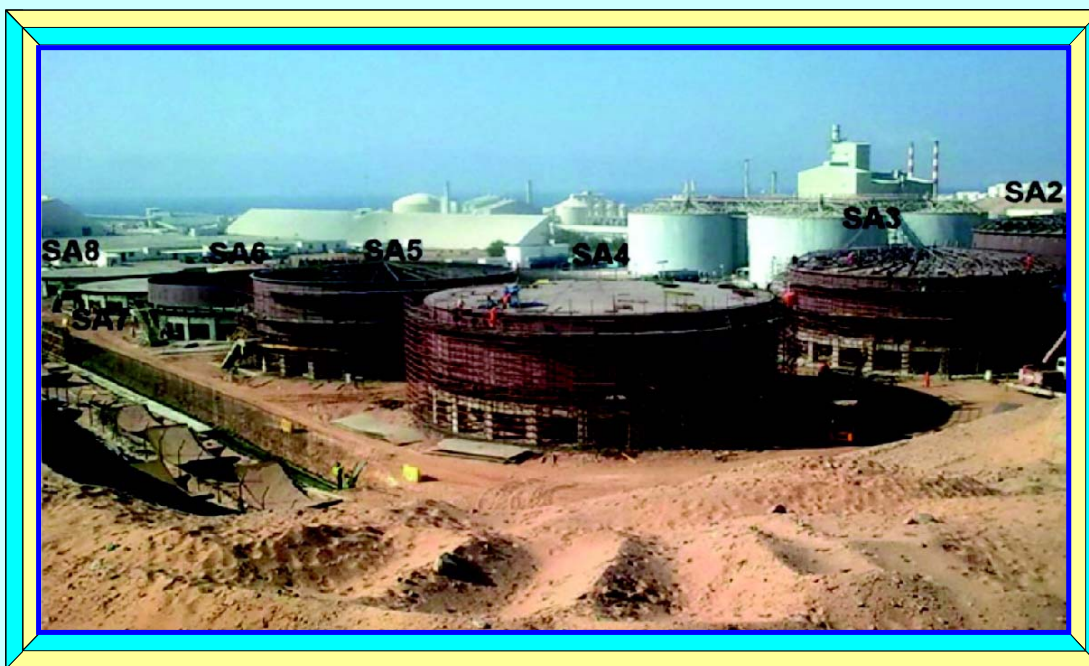
JIFCO, Jordan Tank Farm Project comprising of 7 nos. of Phosphoric Acid Tanks each of 10,000 Ton capacities at Jordan.
