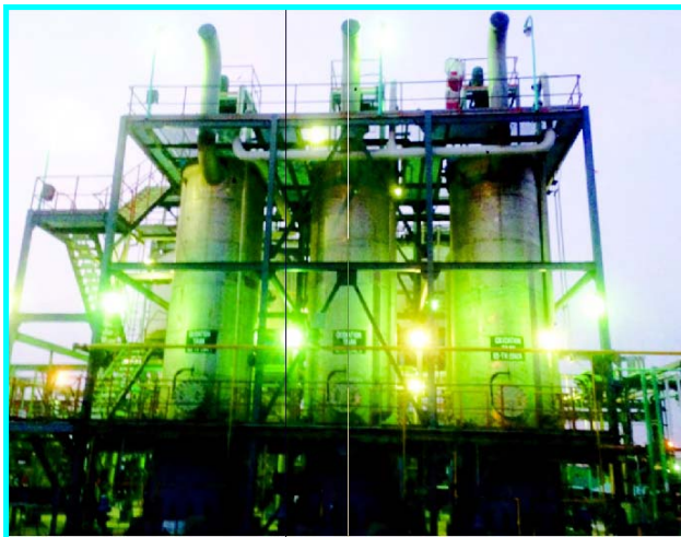
A View of Oxidation Tank (PTU) at HPCL Visakh Site
