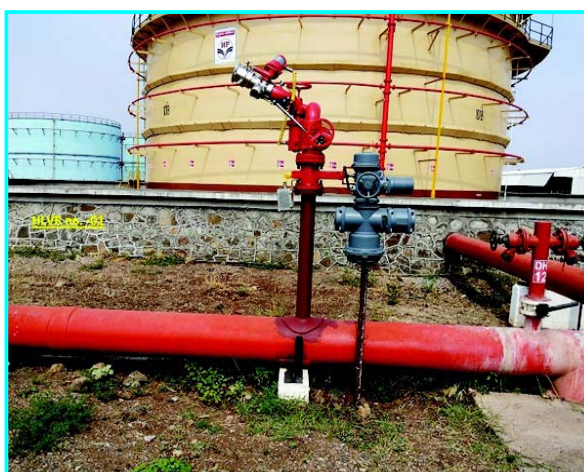
PMC services for HPCL Terminal Automation
