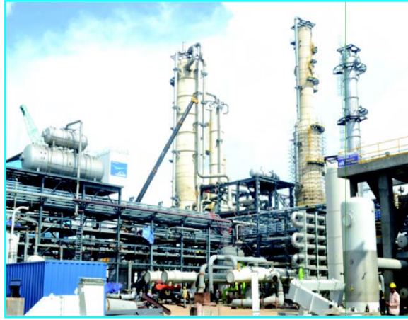
20,000 TPA Hydrogen Generation Unit at Barauni Refinery for IOCL
