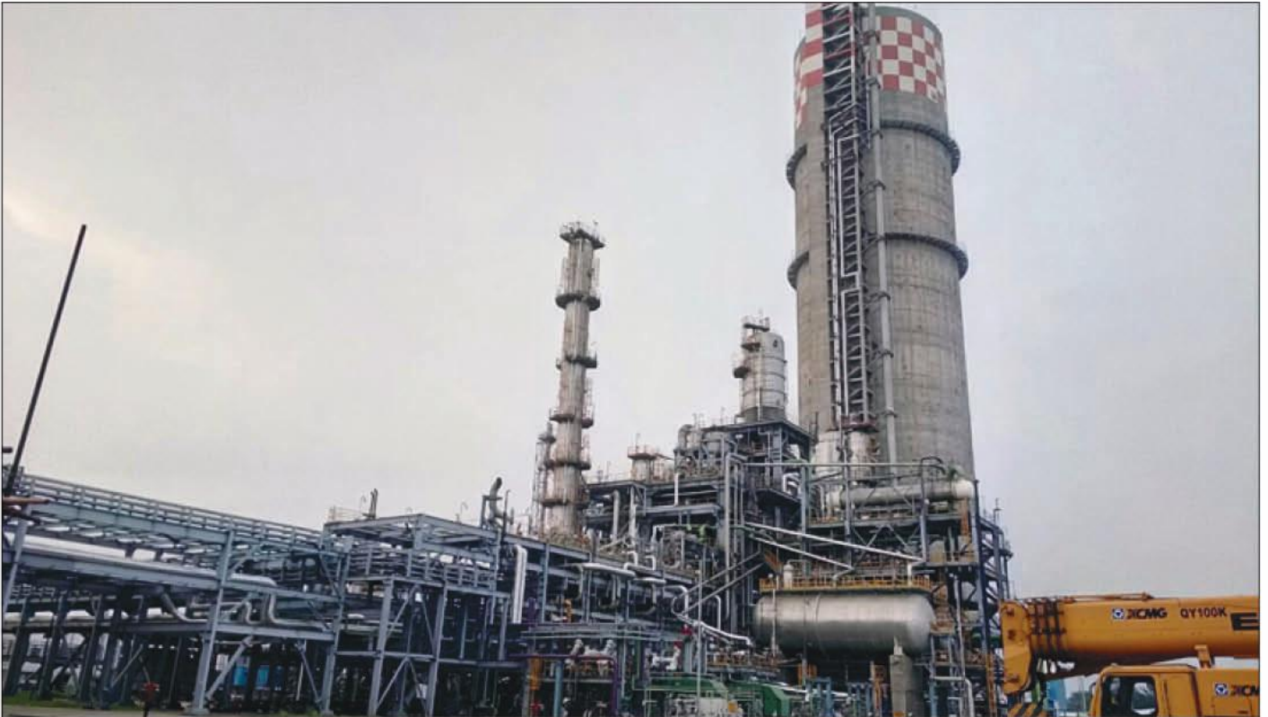
A view of Matix Fertilizers plant executed by PDIL.
