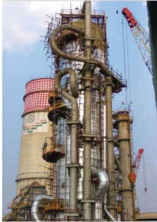
A VIEW OF HP-LP VESSEL AT IFFCO PHULPUR
