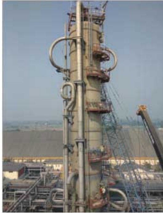
A VIEW OF HP-LP VESSEL AT IFFCO PHULPUR
