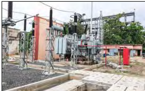
TFL -Electrical Substation for Const. Power
